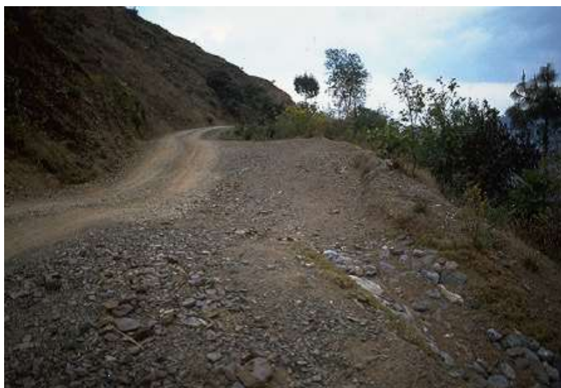
Figure 69: Rolling dip on a rural road with inslope section 41
