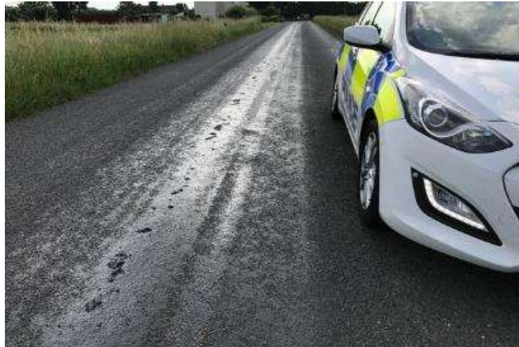
Figure 38: Road in Cambridge shire, United Kingdom with melting asphalt in June 2017 19
