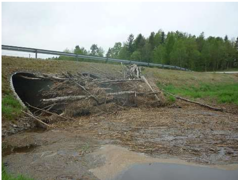
Figure 93: Culverts in Sweden blocked by trees and debris 63
