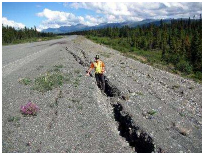
Figure 53: Cracks from melting permafrost at the embankments of the Alaska Highway 31
