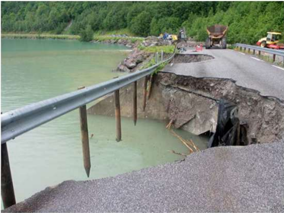
Figure 88: road in Norway destroyed due to erosion caused by a flood. 58
