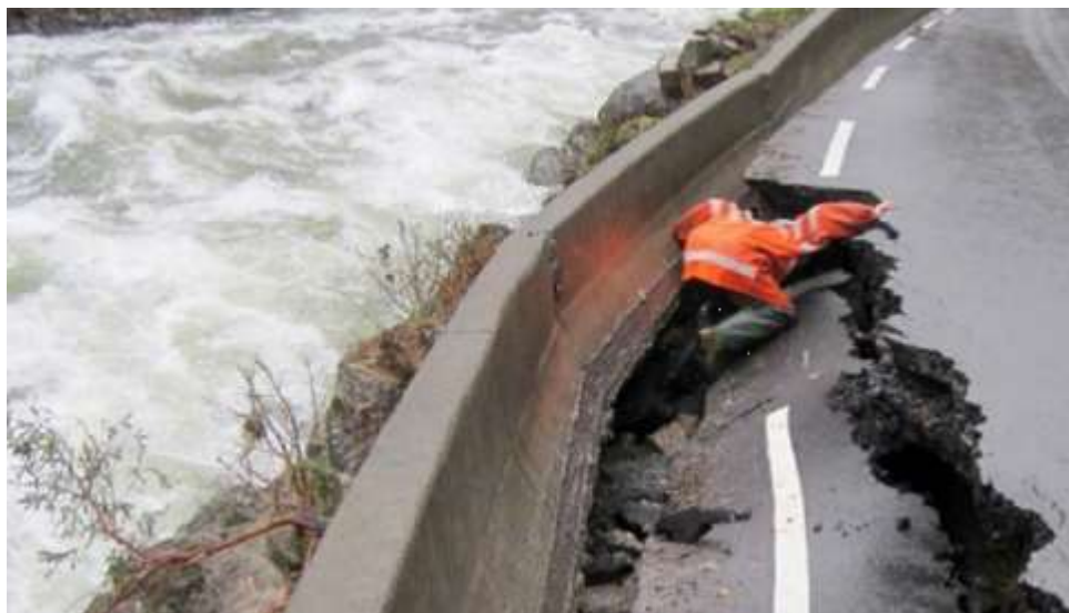
Figure 89: partly collapsed road after flood caused damages of the earthwork 59
