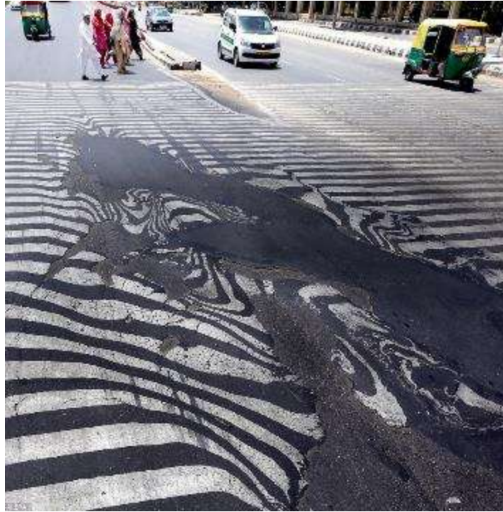
Figure 37: melting asphalt road in India in summer 2016 18
