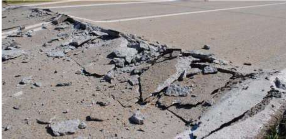
Figure 79: Blow up at a concrete road in Austria 50
