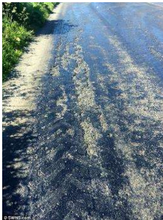
Figure 39: Rural road in the UK with melted pavement 20
