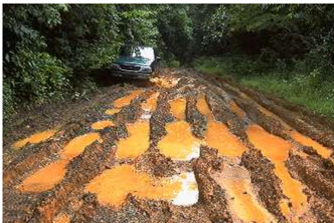
Figure106: unpaved road in Central America destroyed by standing water 70
