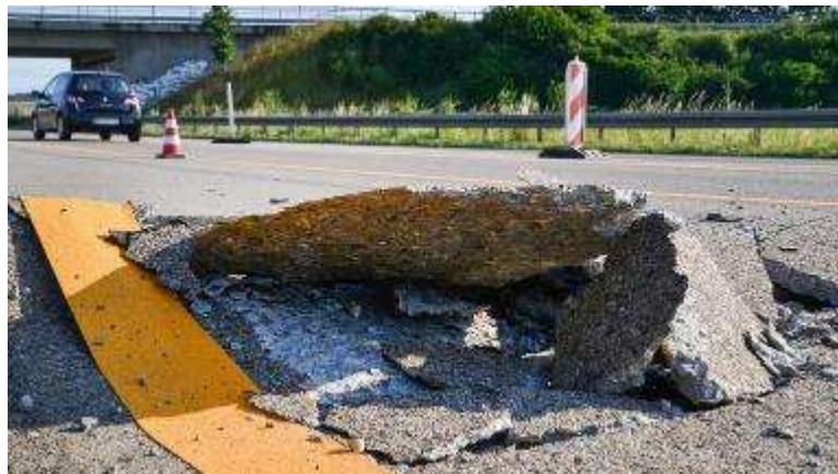
Figure 80: Blow up at a concrete road in Austria 51
