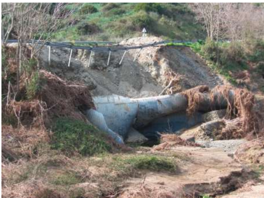
Figure 54: Collapsed culvert in Sardinia with a damaged earthwork 32
