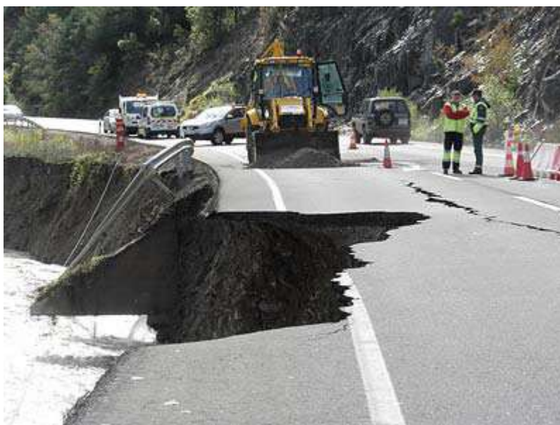
Figure 87: road in Spain destroyed due to erosion caused by a flood 57
